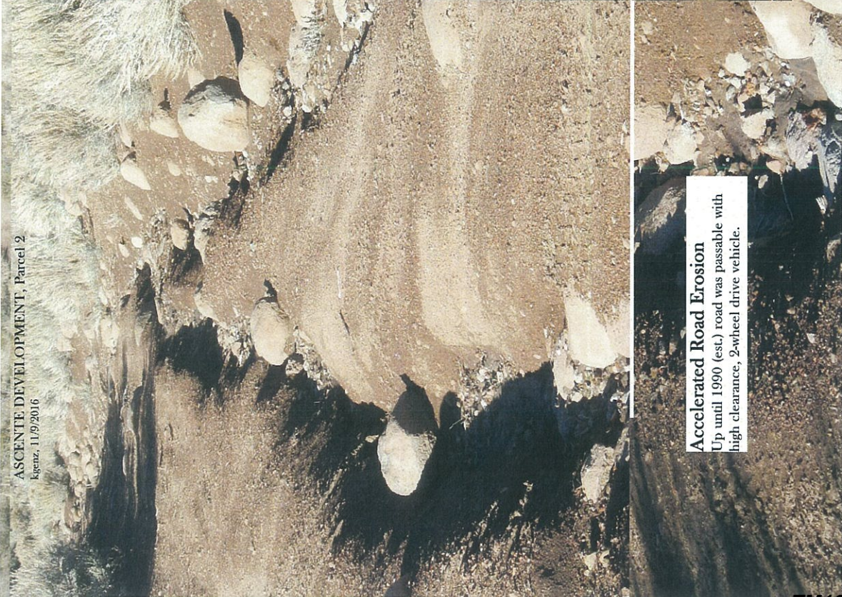
Accelerated Trail Erosion Trail was built to install utility line.
