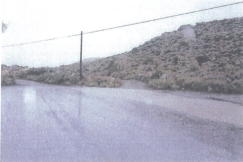
P2. Storm water draining onto Cedarwood Dr.
